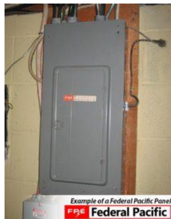
Federal Pacific Electric (FPE) circuit breaker panel
